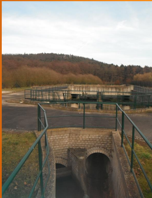
Photo. Rainwater treatment facility, Prague
